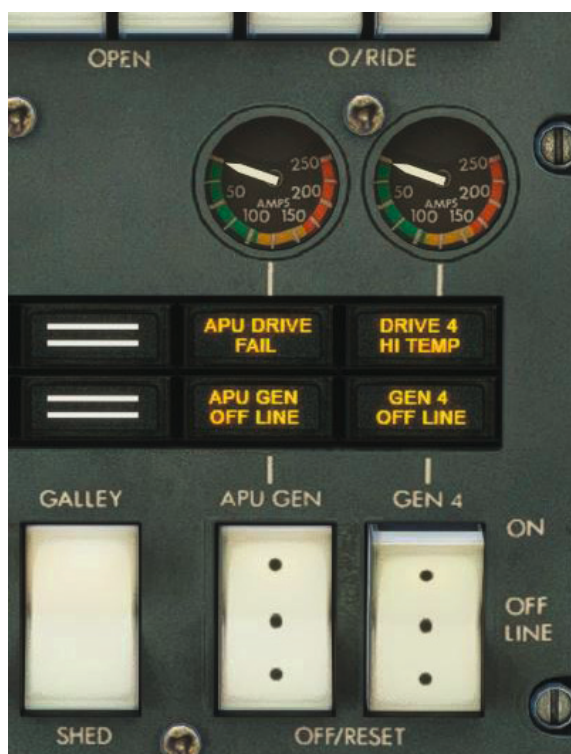
Electric panel – overhead
